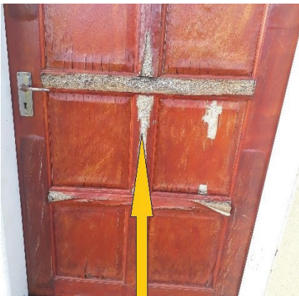
Door in poor condition
