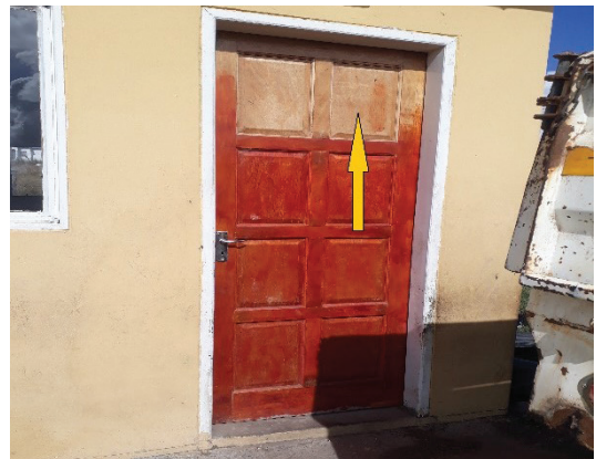
Door not fully painted
