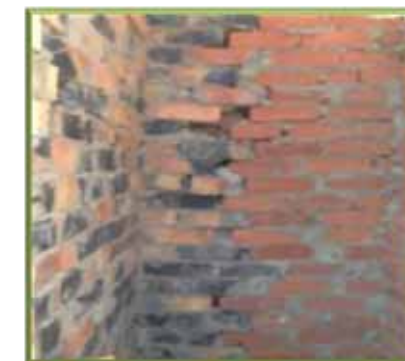
Picture 12: Internal walls with poor brickwork
