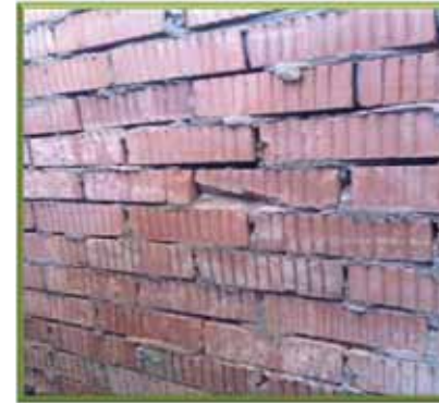
Picture 17: Walls with poor brickwork
