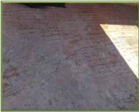
Picture 13: Stress cracks in walls
