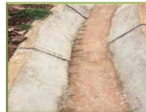
Picture 10: Exposed rebar on storm water structures
