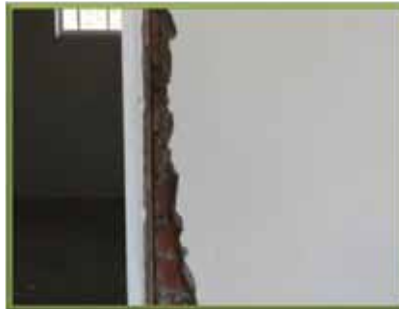
Picture 2: Cracked light screen door
