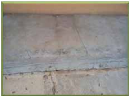
Picture 3: Cracks visible on apron
