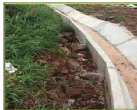
Picture 9: Unsupported storm water structures
