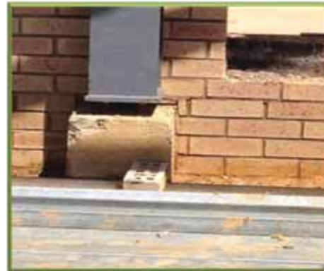
Picture 16: Steel column dangling above its plinth
