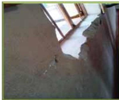
Picture 4: Plaster cracking around windows
