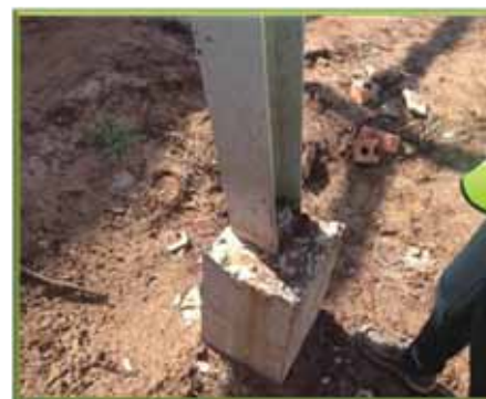
Picture 11: Steel column is off-centre on its plinth
