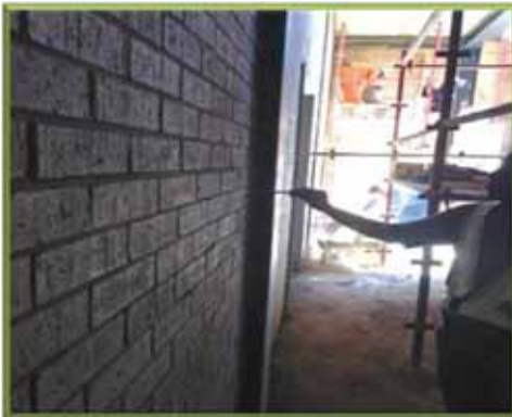
Picture 15: Door frame showing skew wall
