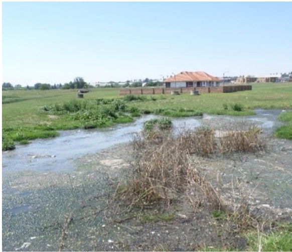
Sewage overflows at Evander wastewater pump station due to vandalism (Govan Mbeki, Mpumalanga)
