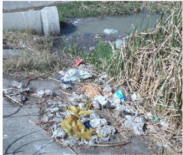
Mothohtlung wastewater treatment works has been completely demolished due to vandalism and theft, but still receives sewage inflows that are discharged without being treated (Madibeng, North West)
