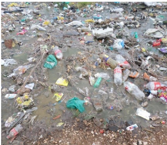
Raw sewage overflows at Boegoeberg wastewater pump station due to blocked manholes (!Kheis, Northern Cape)
