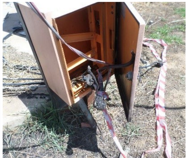
Brandfort wastewater treatment works has totally collapsed and been non-functional for years due to vandalism and stolen equipment (Masilonyana, Free State)
