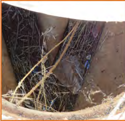
Picture 2: Debris in the dry unused manholes
