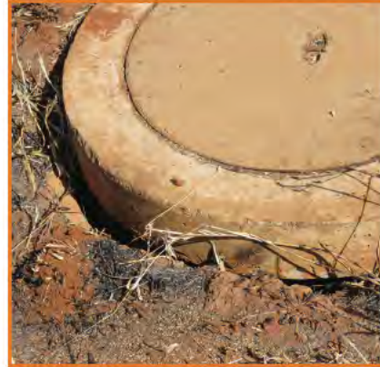
Picture 3: Manholes starting to deteriorate
