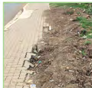
Picture 28: Deformation of paving
