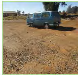
Picture 35: Poor grading and finishing
