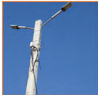
Picture 16: Vandalised wiring
