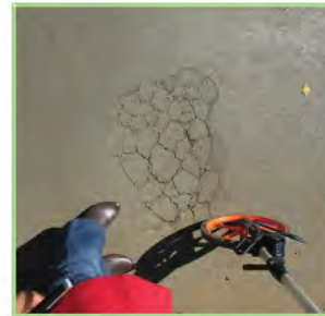
Picture 20: Sign of distress
