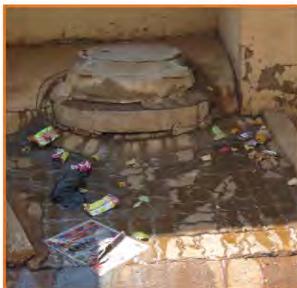
Picture 18: Raw sewage flowing from a manhole
