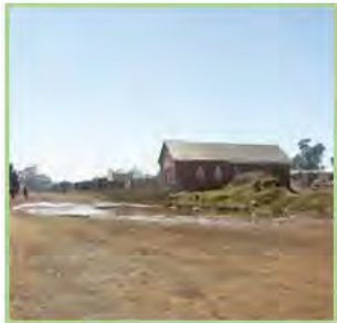
Picture 33: Ponding water on gravel road
