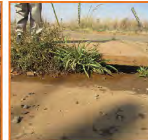
Picture 5: Sunken and partially blocked kerb inlet
