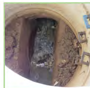
Picture 30: Solid waste thrown into open manholes
