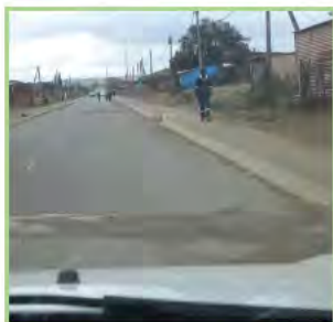
Picture 27: Poorly constructed speed hump
