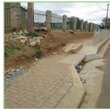
Picture 23: Blocked kerb inlet
