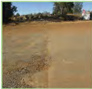
Picture 34: Poor construction of surface joint
