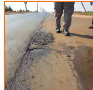
Picture 4: Poor patch repair and pothole
