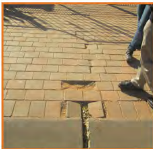
Picture 11: Poorly reinstated paving
