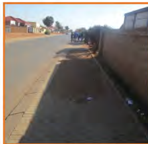
Picture 12: Missing paving
