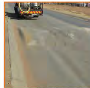
Picture 7: Mechanical damage on speed hump
