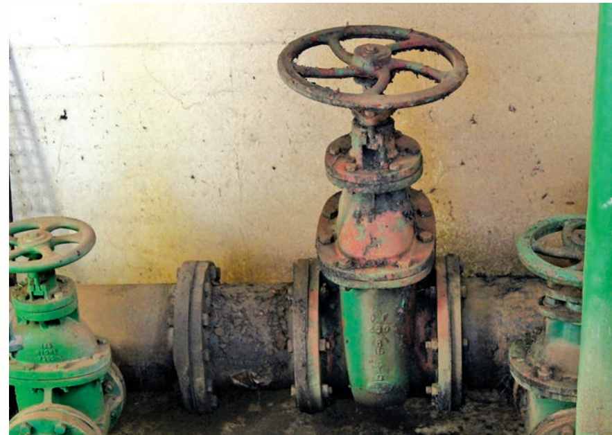
Picture 6: Condition of infrastructure without required inspection and maintenance
