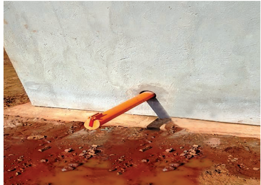
Picture 4: Leaking valve resulting in a waste of water
