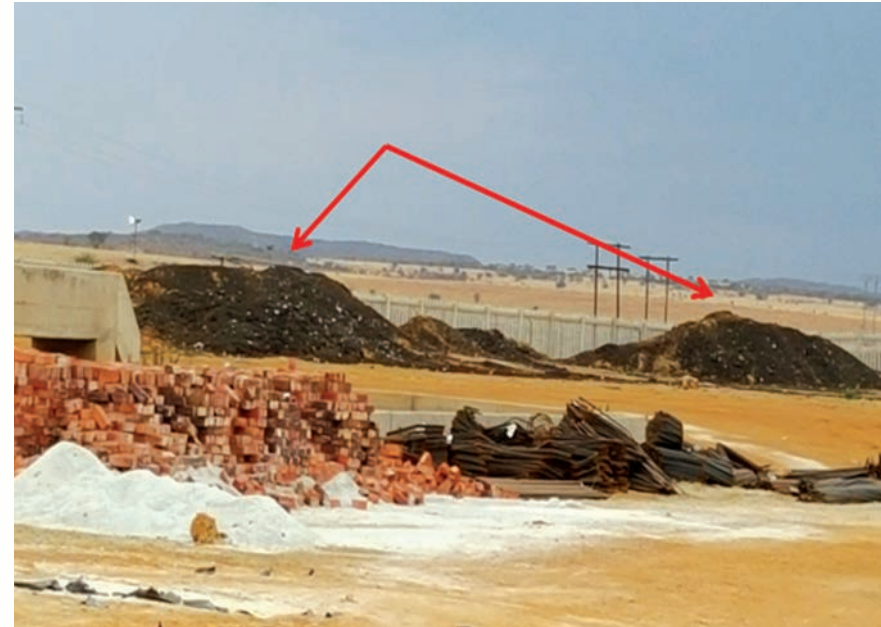
Picture 2: Dried sludge (by-product) not disposed of was accumulating on site at the existing Maquassi WWTW
