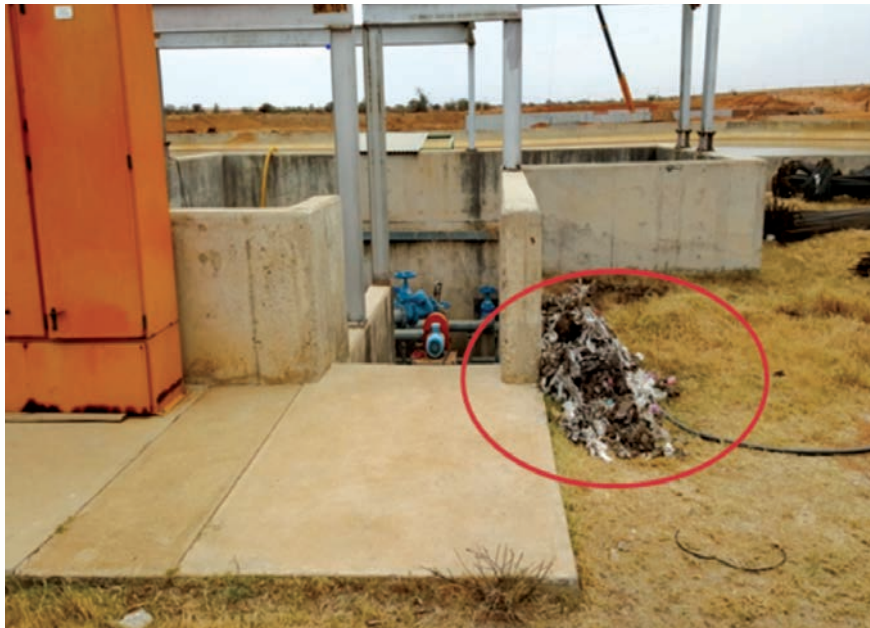
Picture 7: Filtered waste material was not disposed of and was left exposed on site (NW)
