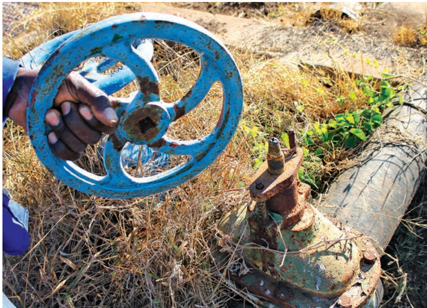
Picture 5: Condition of infrastructure and extent of disrepair
