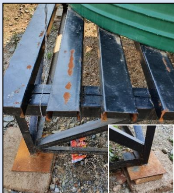
Steel stand for water tank at Asibemunye Secondary School corroded and not level. with wood used to stabilise (inset)
