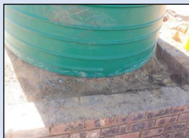
Gauteng: Boitumelo (no concrete slab)
