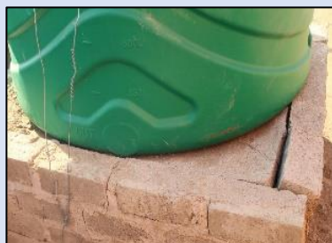
North West: Bojanala - Letlhabile G (cracked platform)
