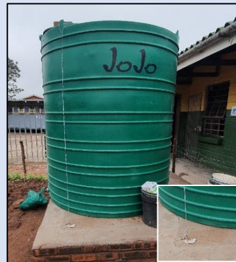
Cracking on concrete structure at Elangabini Junior Primary School
