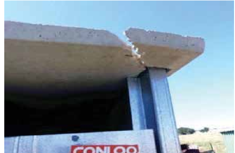
Picture 6: Roof damaged
